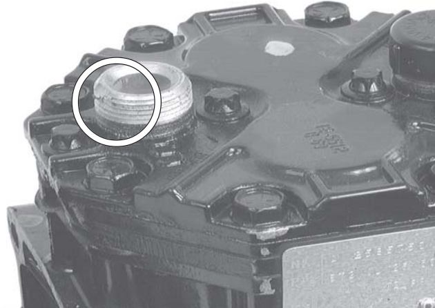
Dropped Compressor shown by the flat dent in threads.
